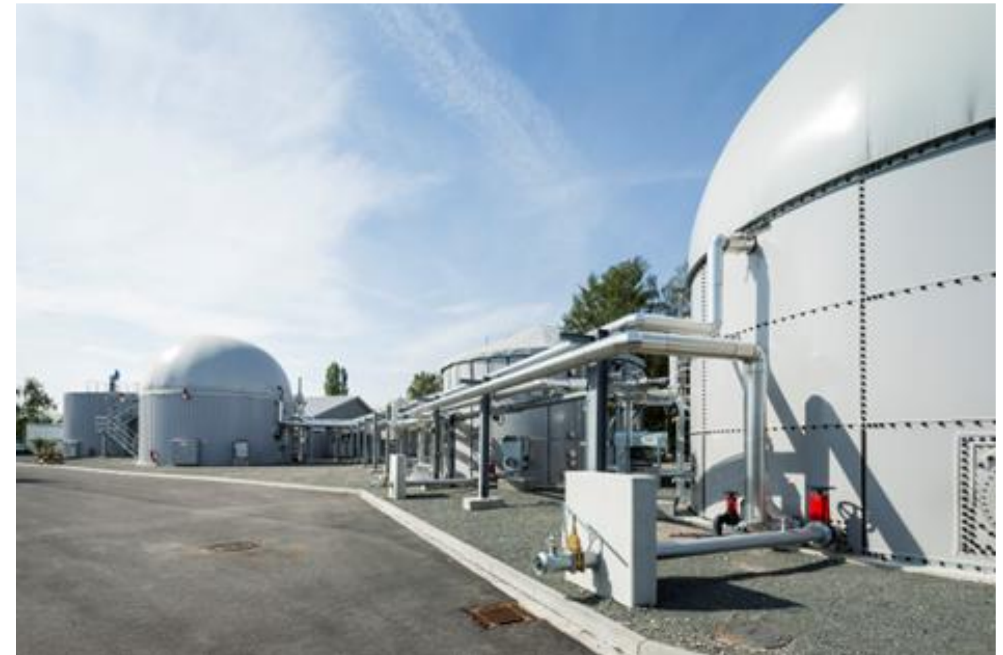
Photo: Biogas research plant at DBFZ
